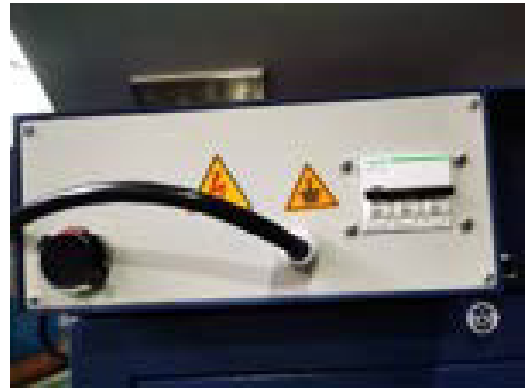
Schneider Power Source
